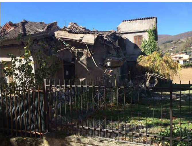
Earthquake damage in Norcia, Umbria
